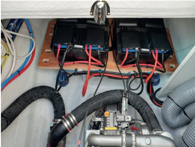
Service battery bank
