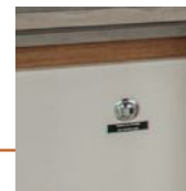
SWITCH Flow time : 15 sec
