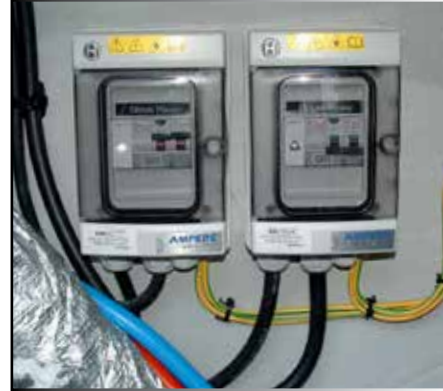
SHORE AIR CONDITIONING + ON-BOARD AUTOMATIC BREAKERS
