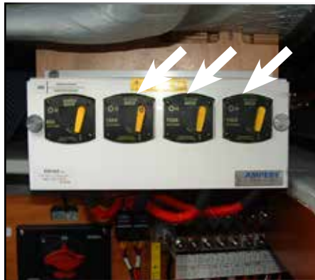
AUTOMATIC BREAKERS FOR THE ELECTRIC WINCHES
