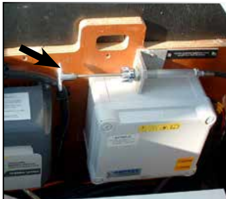
TANK / GENERATOR SELECTION PULL ROD
