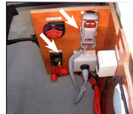
WINDLASS CONTROL + AUTOMATIC BREAKER
