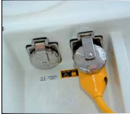
ON-BOARD + AIR CONDITIONING SHORE POWER SOCKETS
