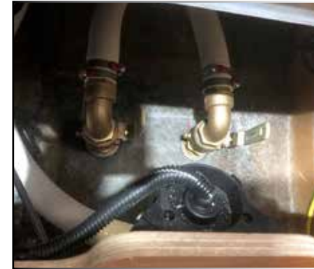
OVERBOARD DISCHARGE VALVES
