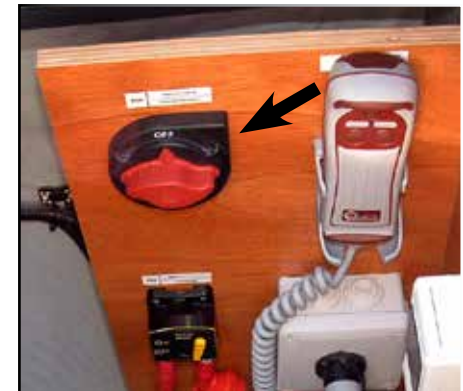
CUTOUT AUTOMATIC BREAKERS
