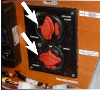
BATTERIES + STARBOARD ENGINE COUPLING CUT-OUT
