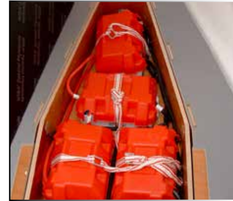
THRUSTER BATTERY BANK
