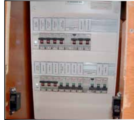
AUTOMATIC BREAKERS BOX (110 V - 220 V)
