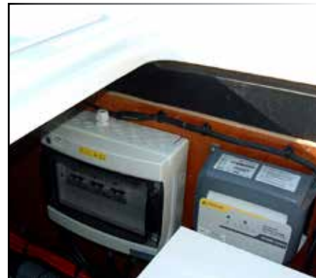
CIRCUIT-BREAKERS + CHARGER AUTOMATIC BREAKERS
