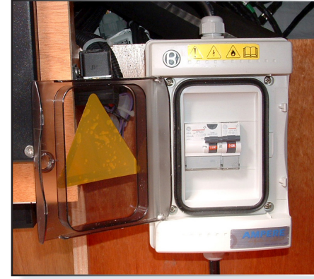
SHORE POWER SOCKET AUTOMATIC BREAKER
