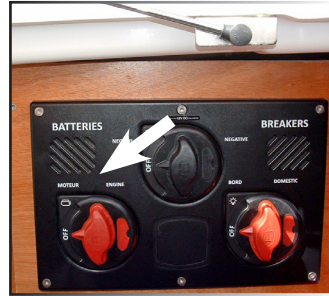
STARBOARD ENGINE CUT-OUT
