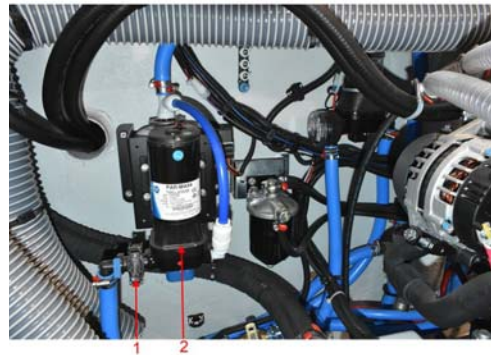
Location: Port engine compartment
