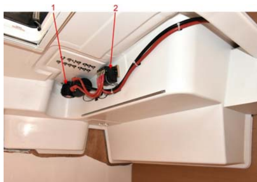
Access: Port and starboard aft cabins
