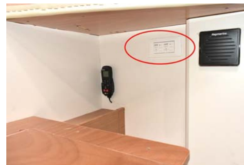
Circuit breaker of sockets Location: Chart table
