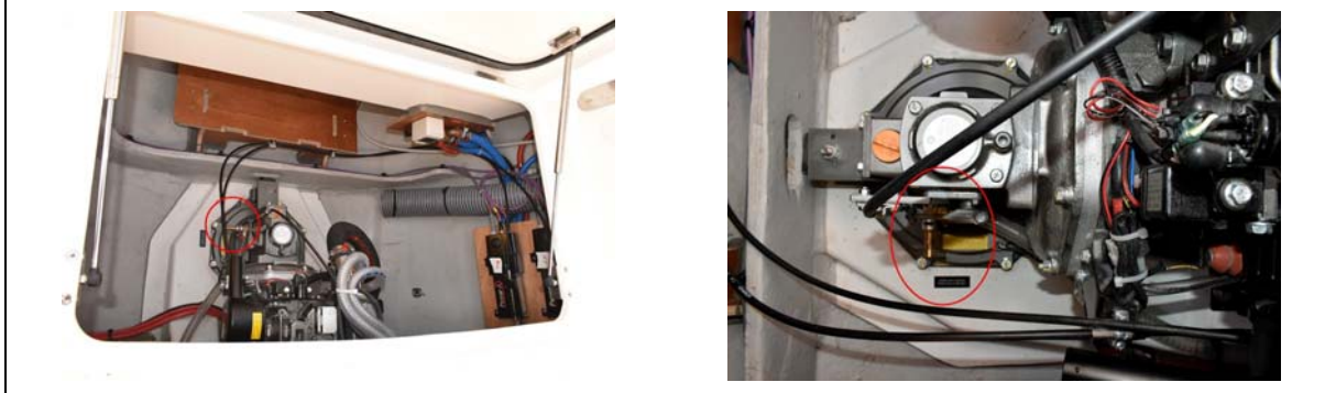
Engine water intake valve: Located directly on the saildrive
