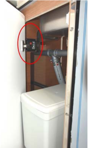
Gas solenoid (US Version) Location: Under the sink
