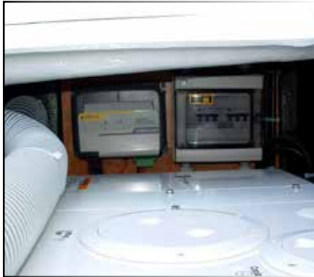
CHARGER + AUTOMATIC BREAKERS OF THE GENERATOR
