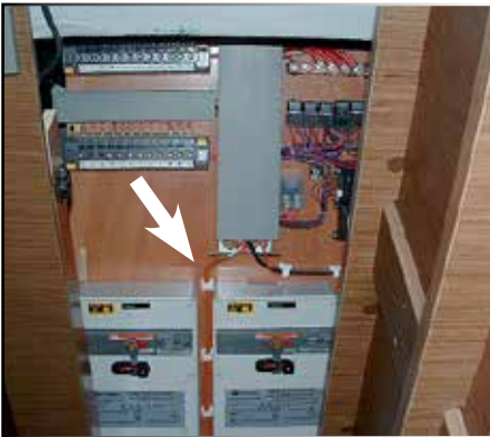
MANUAL SELECTOR SWITCHES
