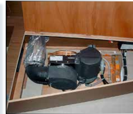
AIR CONDITIONING UNIT
