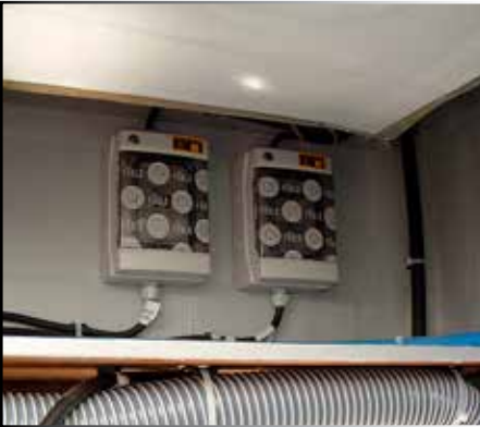
SHORE POWER SOCKETS CIRCUIT BREAKERS
