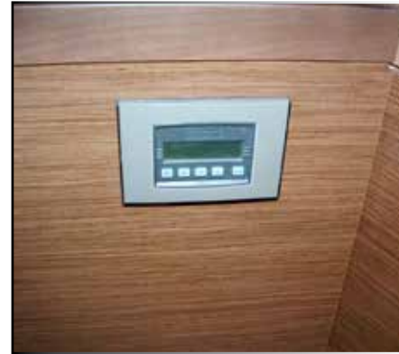
AIR CONDITIONING CONTROL
