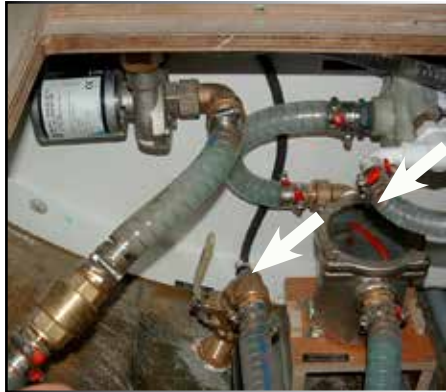
VALVE + WATER FILTER OF THE GENERATOR
