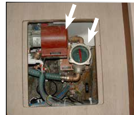
SEA WATER PUMP + FILTER
