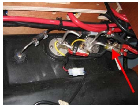
Fuel supply valve: located directly on the tank
