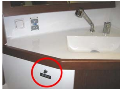
Control - Draining pump for shower
