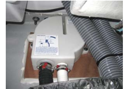
Water - Gas separator
