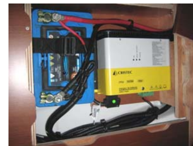
Generator battery - 50A Charger - Generator battery
