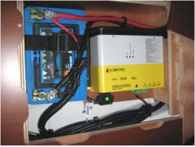
Battery - 50A + Battery charger
