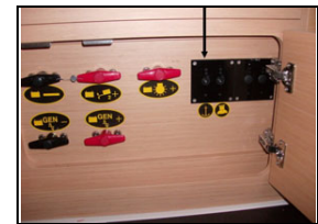
WINDLASS CIRCUIT BREAKER - 100A (STARBOARD AFT CABIN)
