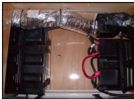
Set - Service batteries 2 x 140A Spare battery 2 x 140A (Reference 2)
