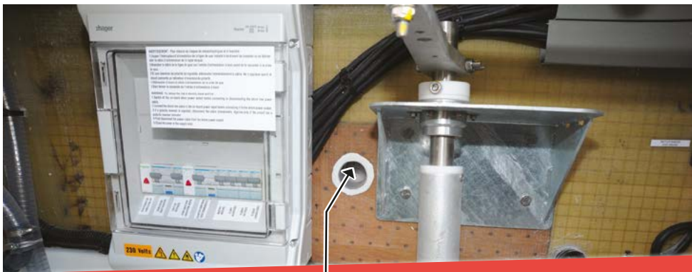
Fire extinguisher outlet in port engine compartment
