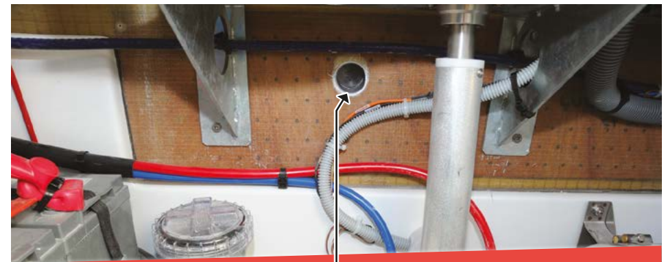
Fire extinguisher outlet in starboard engine compartment
