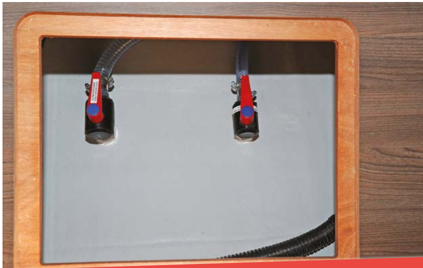
Seawater intake valve
