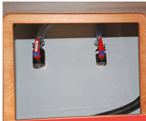
2 Seawater intake valve
