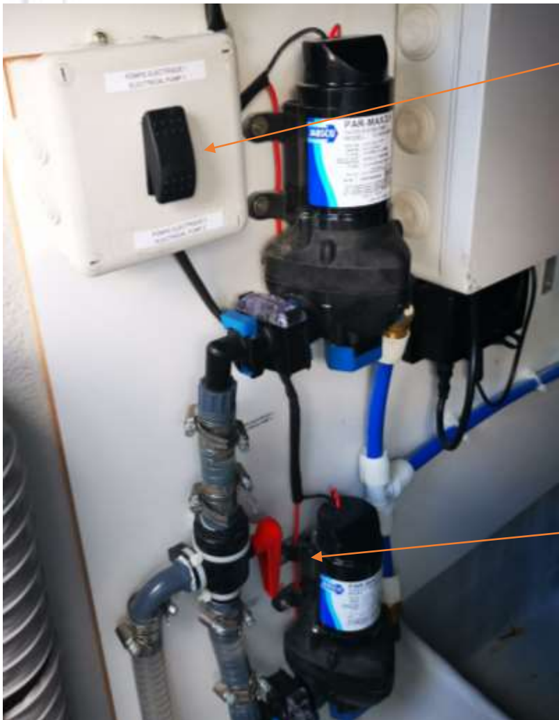
Selector switch for freshwater pumps
