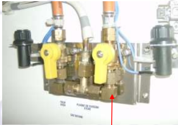
Gas shut off valves under sink
