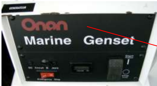
Main breakers for the generator
