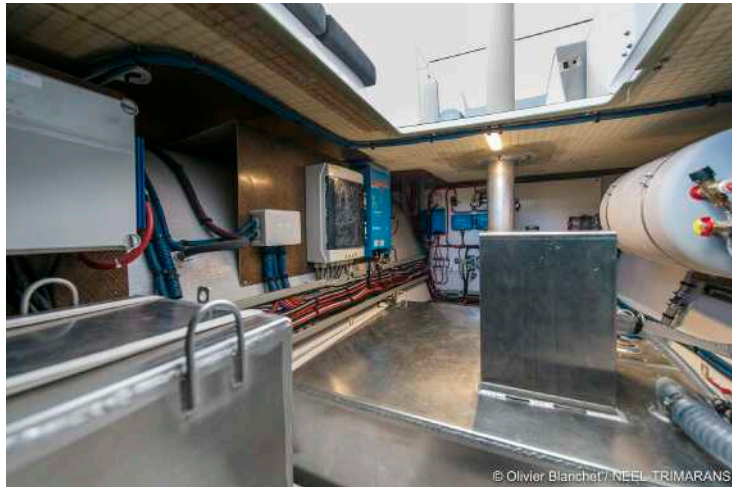
Engine bay with direct access from the technical area
