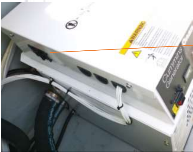
Generator Reset Breaker
