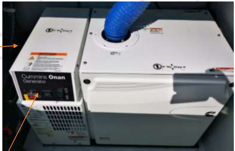
Cummins Onan Generator
