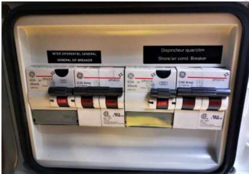
Main shore power breakers in port engine room
