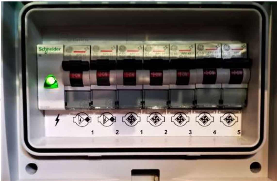
Air conditioning breakers in STBD cabin behind sliding door
