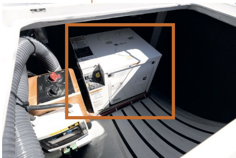
[Option location: starboard forward compartment] [Generator on the picture]
