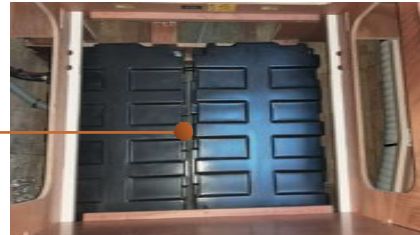
Service battery bank
