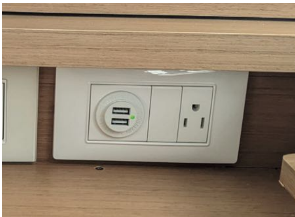
[110V sockets on the picture]
