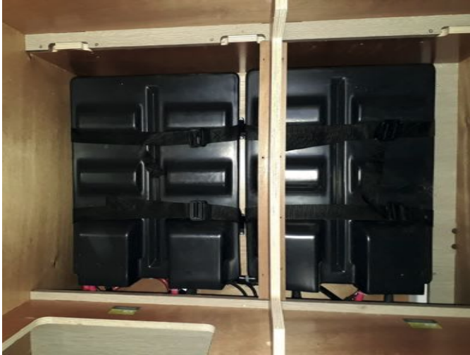
Service battery bank
