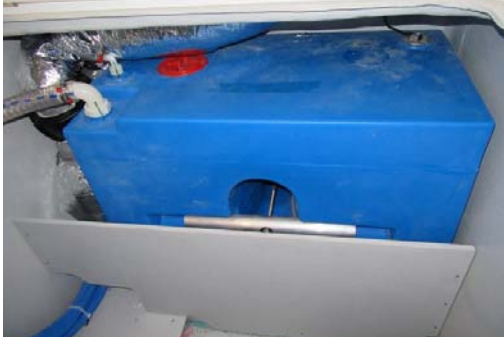
Water tank Location: Locker forward
