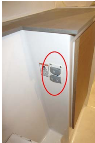
Electric toilet control
