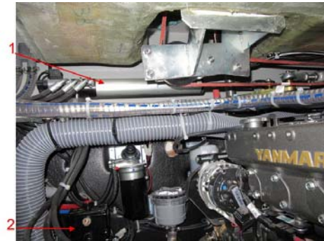
Location: Port engine compartment
