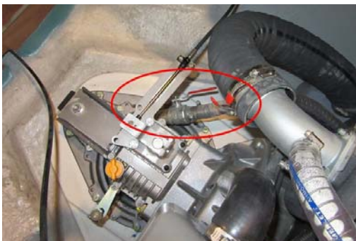
Engine water intake valve: Located directly on the saildrive
