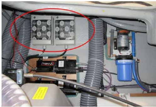
Ref 2: Bipolar circuit breaker (Protection) Location: Starboard engine compartment
