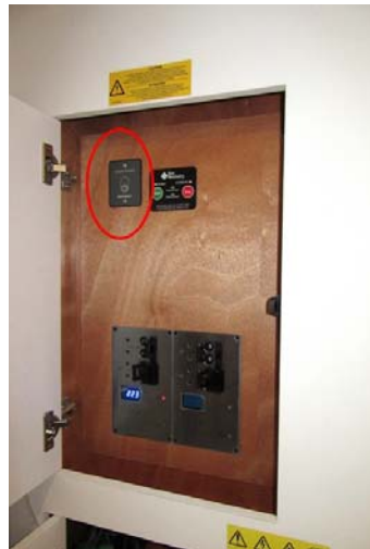
Remote control Location: Port passageway
