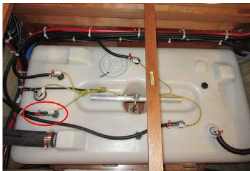
Fuel supply valve located directly on the tank
