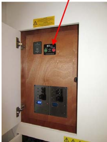
Control panel Location: Port passageway
