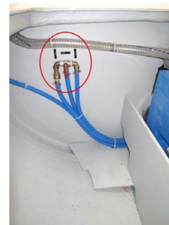
Emplacement of the sea water/fresh water selector valve: Locker forward
